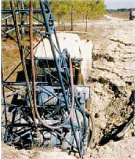
Shallow drilling rig collapsing in to sinkhole
